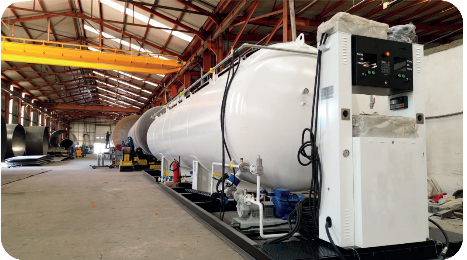
30m 3 LPG Skid Sistem / LPG Skid System
