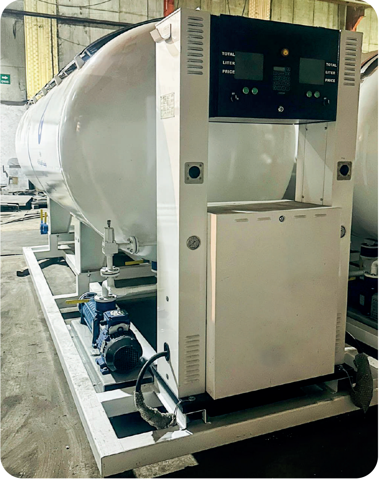
10m 3 LPG Skid Sistem / LPG Skid System
