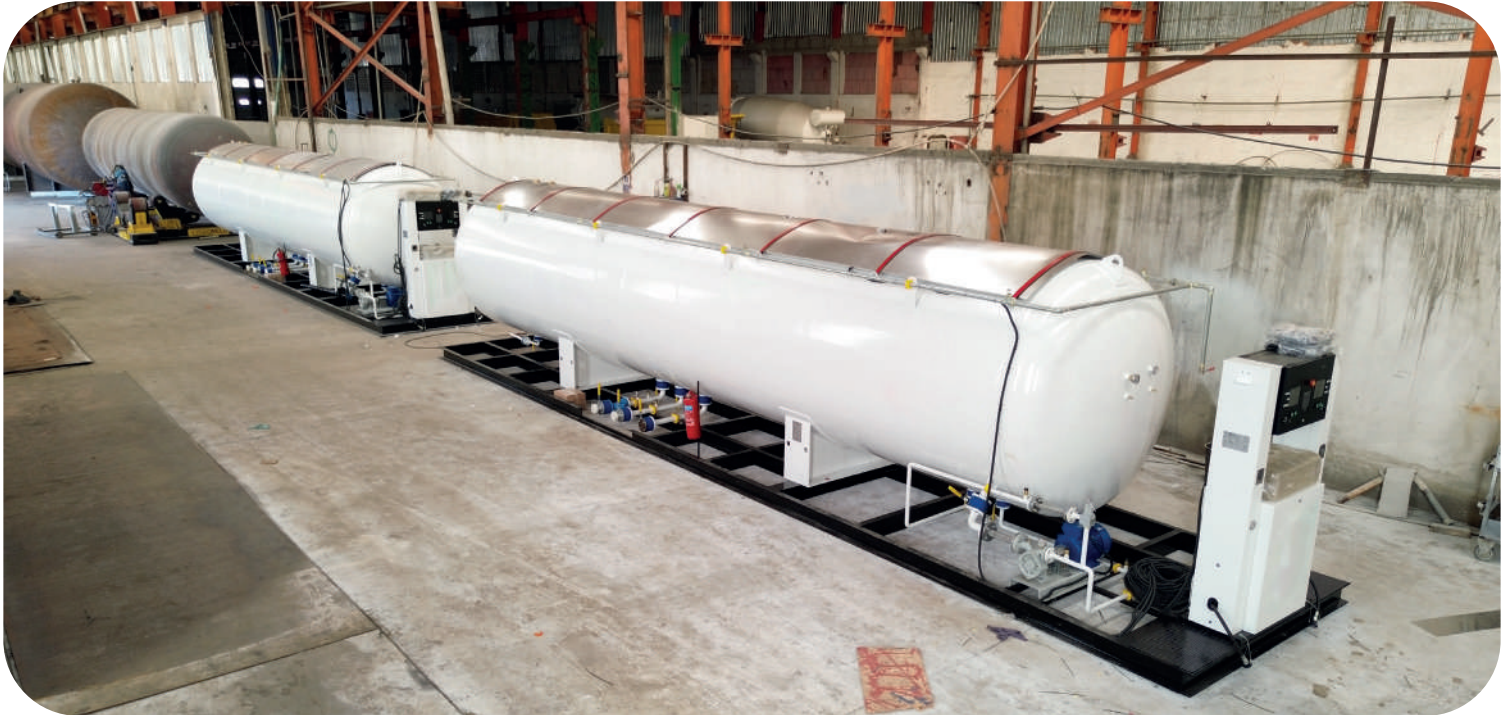
30m 3 LPG Skid Sistem / LPG Skid System
