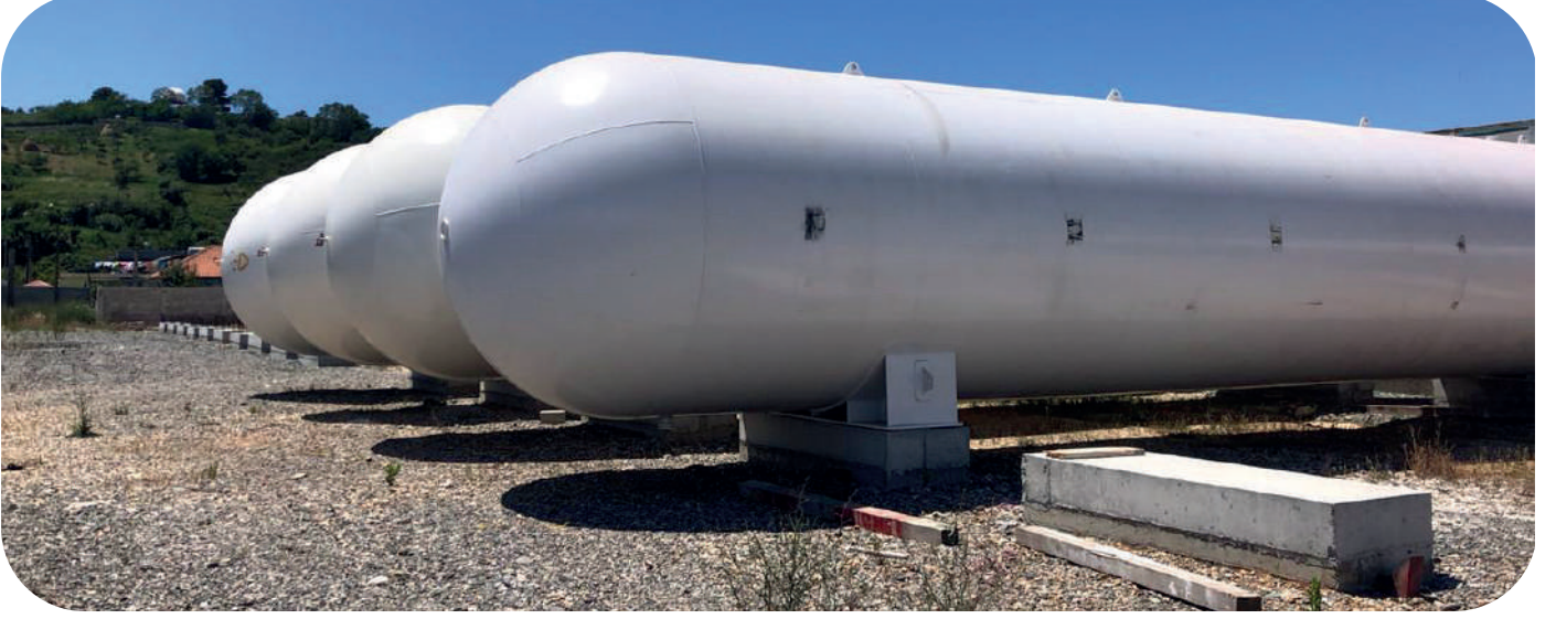
100m³ Stok Tankı / Storage Tank
