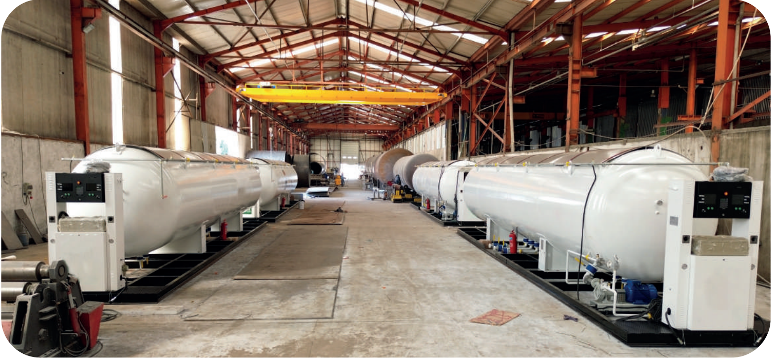
30m 3 LPG Skid Sistem / LPG Skid System
